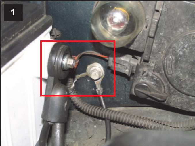
RH Side Battery Ground, Fender Ground G101 (large wire) and possibly G105 (small wire). Doubt small wire is G105.
